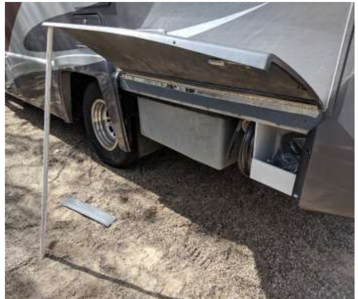
While the paint was curing, I had to mount the larger panel section to a piano hinge so it could be opened for access.
